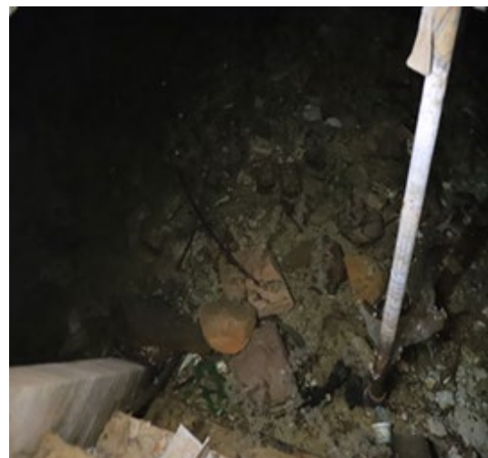
Fig. 6. Showing Ground water inside Nujoumi Dome.
