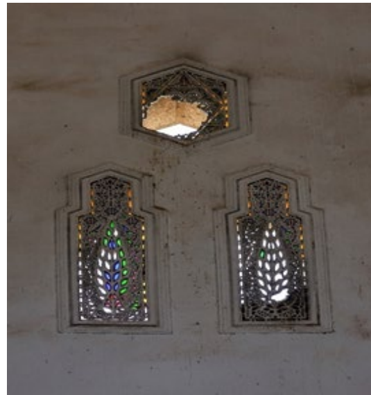
Fig. 8. Shows Deterioration of gypsum window and Qamariyat, and some parts of the decorative elements were lost.
